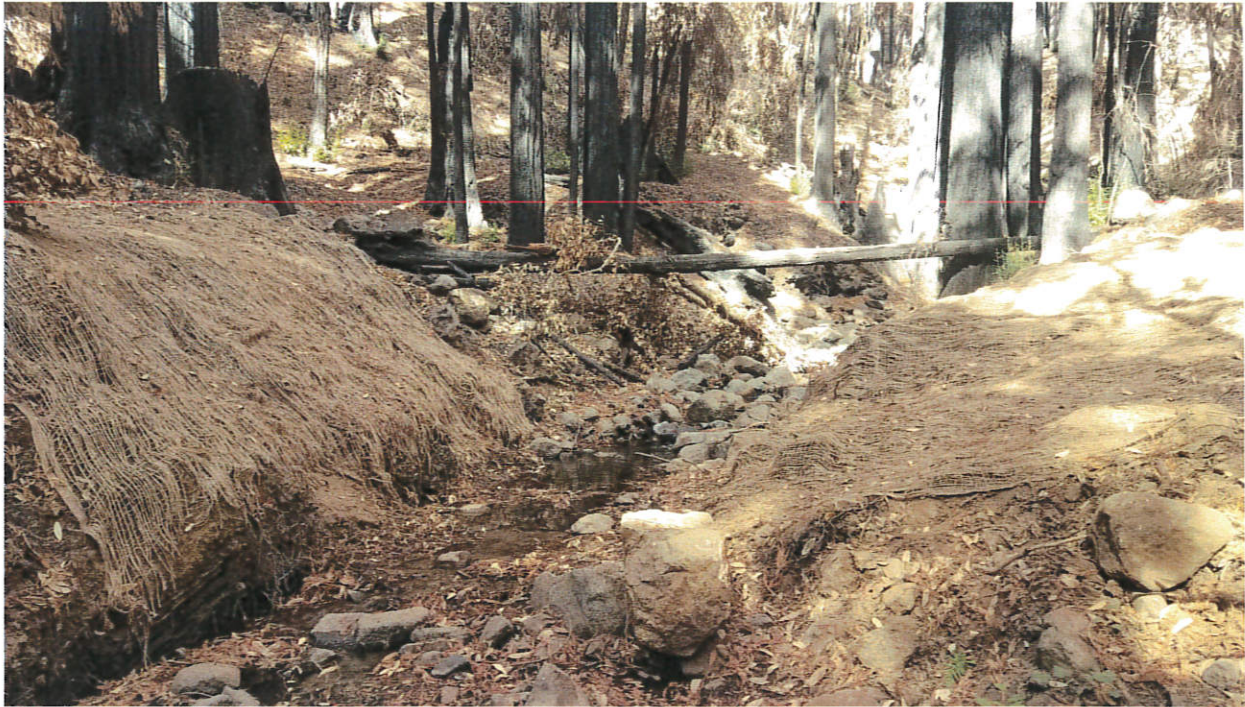
Photo taken 11-6-2020 by R. Sampson. Photo point RS-4. Shows tractor crossing of San Vicente Creek after previous corrective work. Note extent of jute netting only 15' each approach and bare soil not covered at base of left (west) approach.
